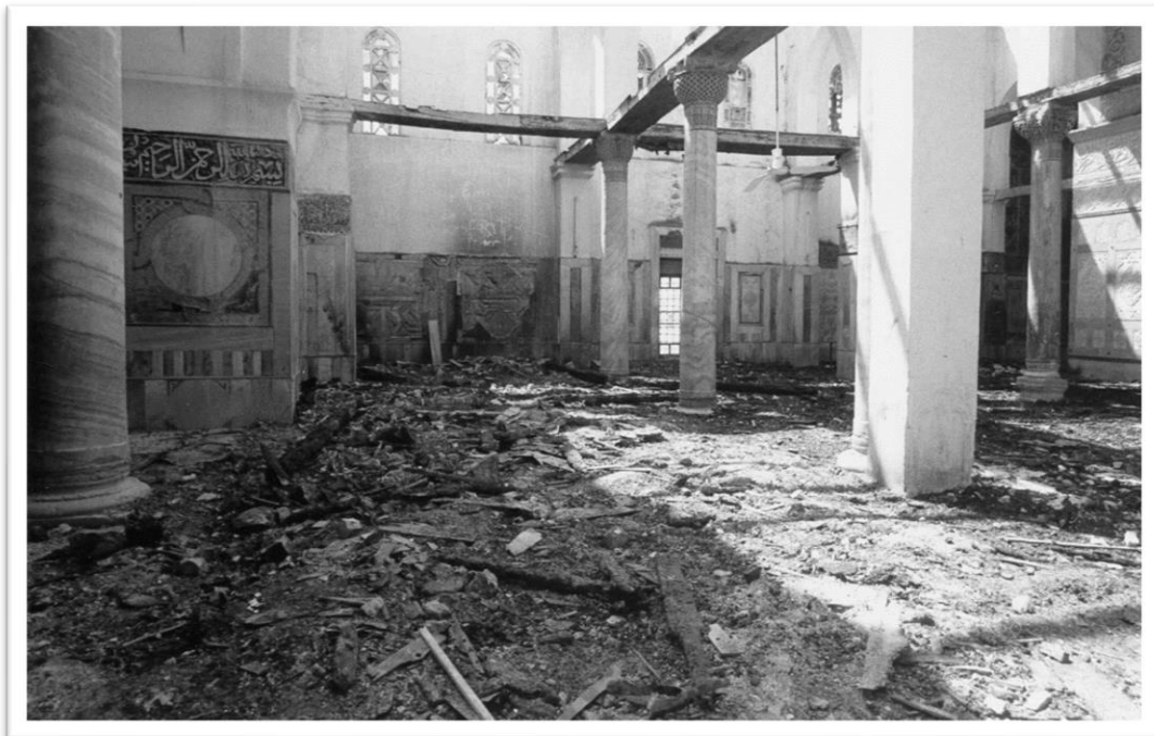
Photo: Damage to the masjid structure and furniture after the fire
